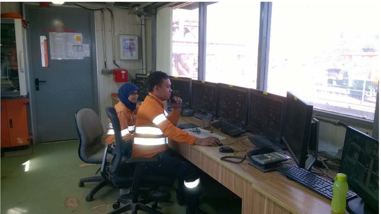
Operators in the processing control room.
